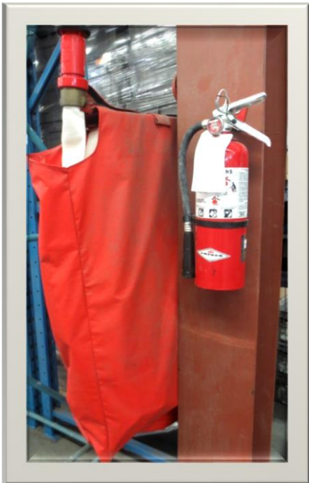
Hose located at front and back of warehouse
